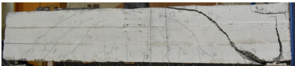
Figure 9: Crack Pattern for Specimen (B-0-2)
